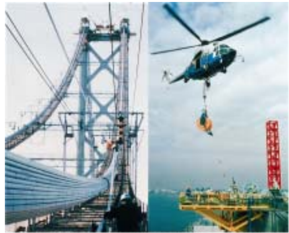
Photo 7: Cable strand construction (left), sea crossing of pilot rope (right) (Akashi Kaikyo Bridge)
