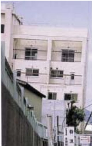
Photo 3: Tilted apartment building
