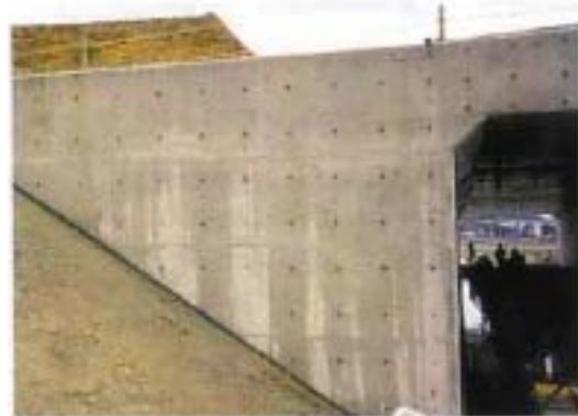
Photo 1: Box culvert prior to the repair
